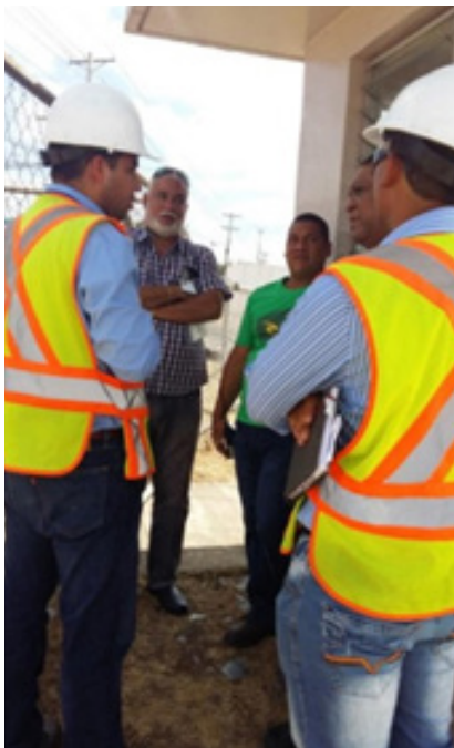
50% of the employees working in the project are from the local communities.
